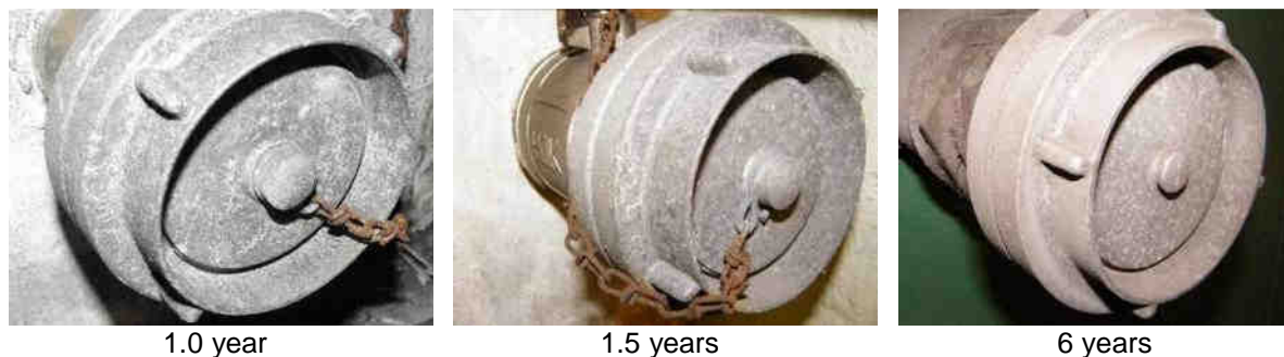
Figure 7: The examples of aluminium corrosion in the tunnels
