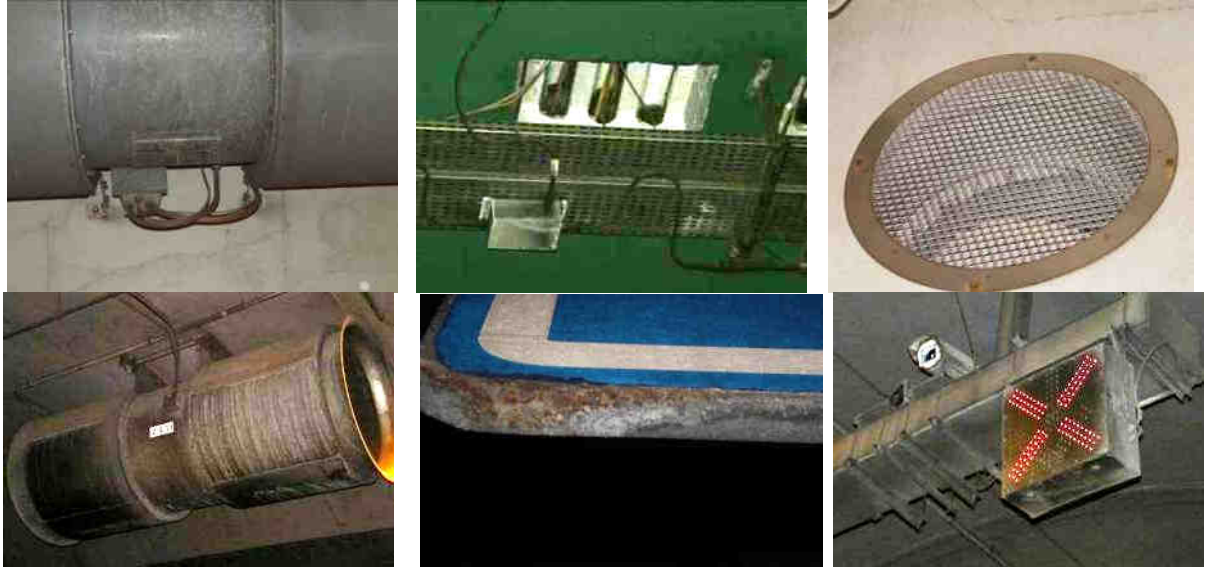
Figure 5: The examples of zinc coatings' corrosion on the tunnel equipments after 1.5 years (above) and 7 years of exposure in tunnels
