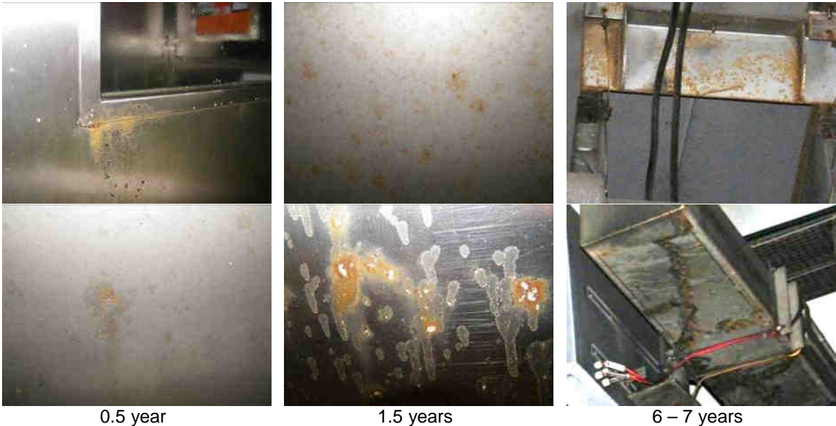
Figure 4: The details of stainless steel corrosion in the tunnels
