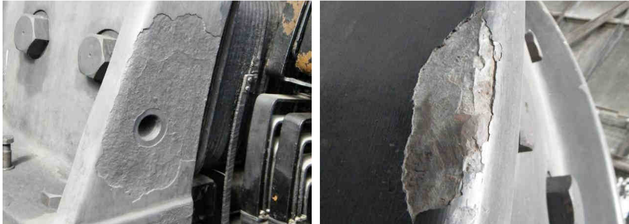
Figure 2: Example of cast iron flaking on machine frames
